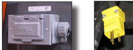
Figure 3-3. AC Outlet and Electrical Plug
