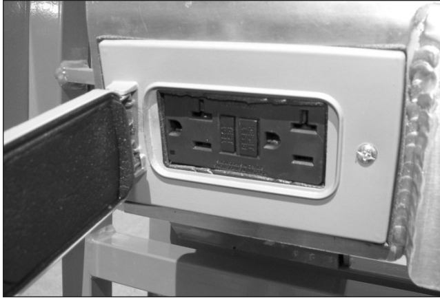
Figure 9.6 – Electrical Power Outlet
